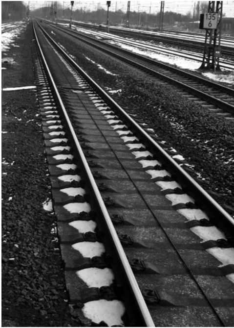
Fig. 1.3 The Rheda system at Rheda station in 2010 (source: Institute of Road, Railway and Airfield Construction, Technical University of Munich)
