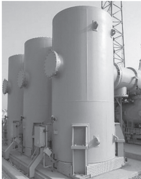
Figure 1.11 Ultrahigh voltage AC tank-type surge arresters in 1000 kV Jindongnan Substation in China.
