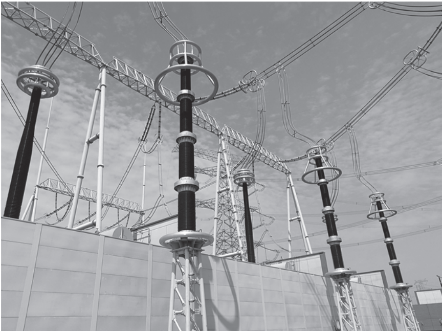
Figure 1.9 1000 kV ultrahigh voltage AC surge arresters with porcelain houses in Dongwu 1000 kV UHV AC substation. Source: Courtesy of X. Zhao.
